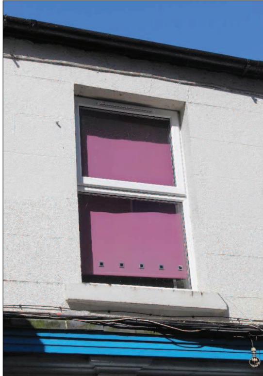
Plate 5. Ruled and lined smooth render to front elevation. Cast iron eaves gutters and heavy window sills with replacement window frames over replacement cornice to timber shopfront.
