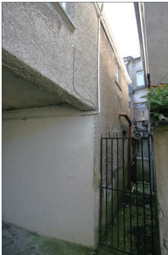
Plate 8. Rear, north elevation of subject property looking towards rear of properties fronting onto Gladstone Street
