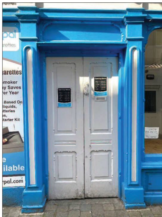
Plate 4. Detail of early to mid twentieth-century main shop entrance doorway with replacement pilaster to west (left) side of opening.
