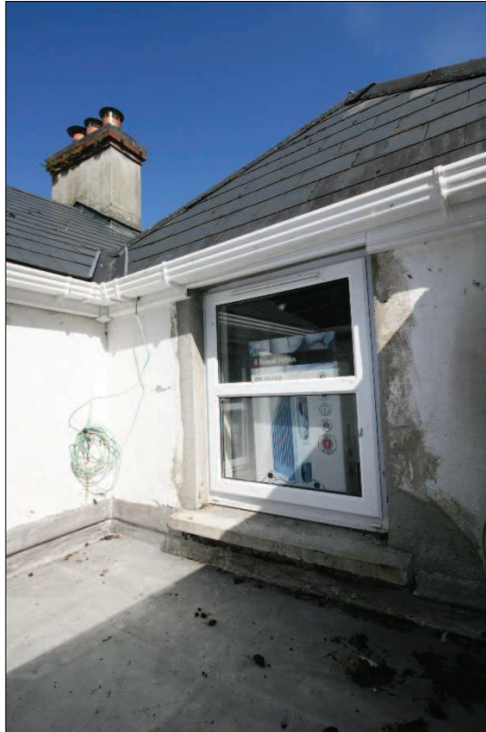
Plate 9. West-facing window at first floor-level overlooking small flat-roofed area between front and rear blocks of subject building.
