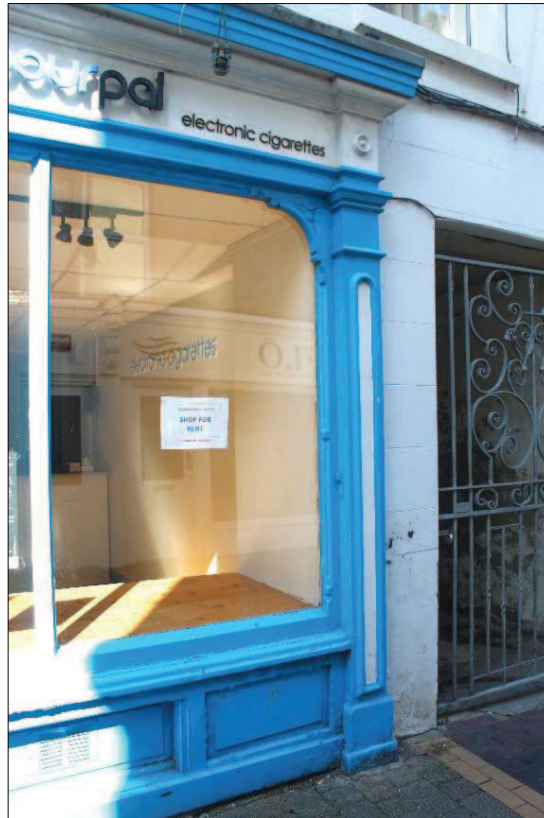
Plate 3. Detail of east pilaster and display window on southern façade. Central glazing bar of display window, shopfront fascia and cornice have been replaced in recent years while many elements of shopfront frame are early to mid twentieth-century in origin.
