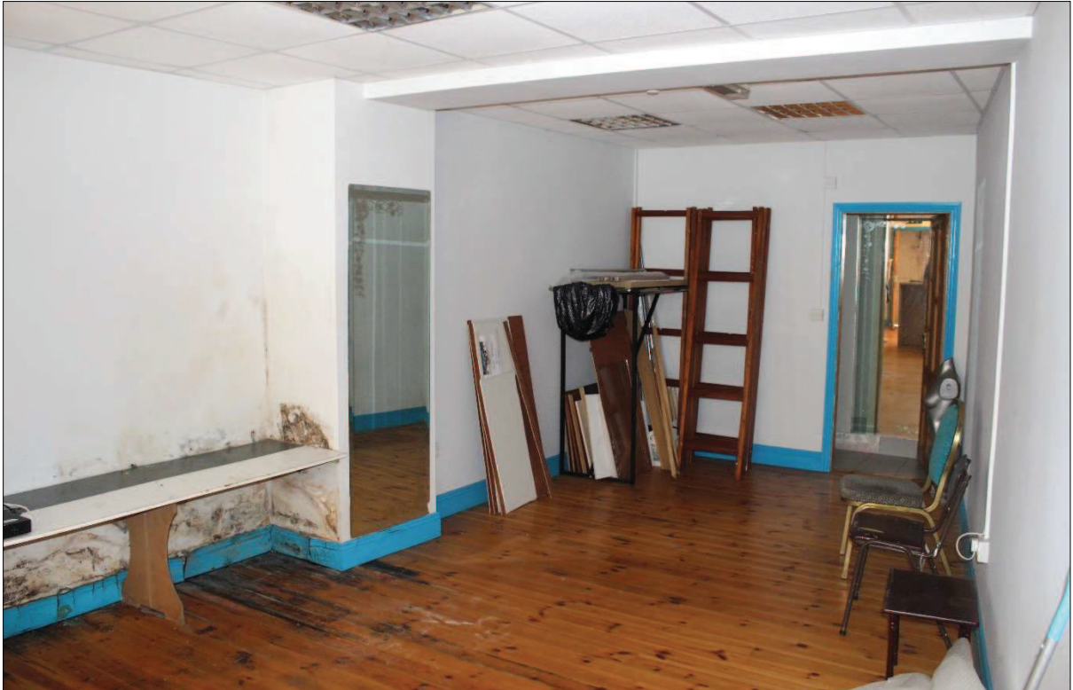
Plate 13. Rear of ground-level shop with partitioned toilet at rear northern end of building. Moisture damage visible to left side of photograph resulted from defect to flat-roofed section above here and has since been repaired.
