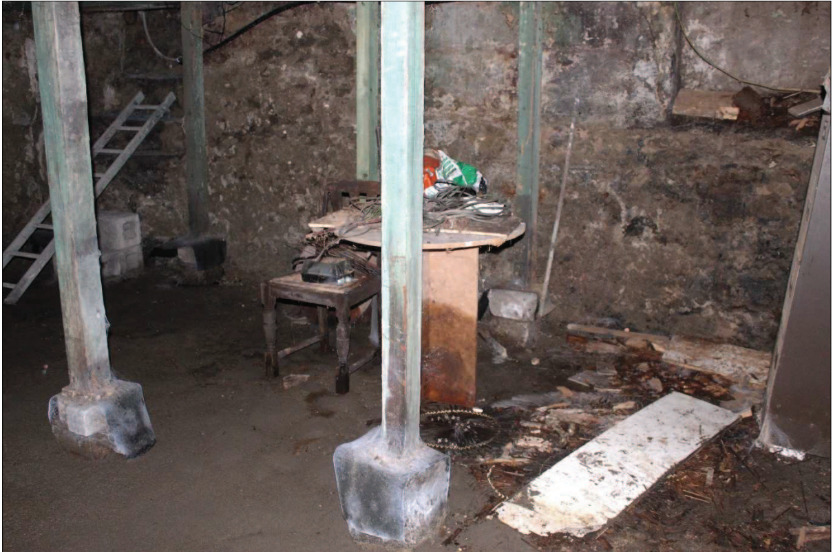
Plate 15. Basement beneath front (south), street-fronting pile of building with earthen floor and blocked front window openings. Floor supports here are treated wood on concrete block supports with PVC damp course beneath wood to prevent upwards migration of floor dampness
