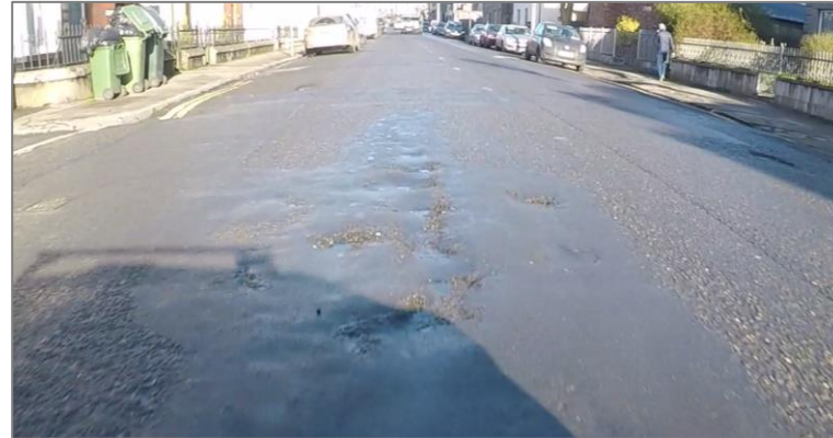
Pavement deterioration (cracking, patching, uneven surface, material loss)
