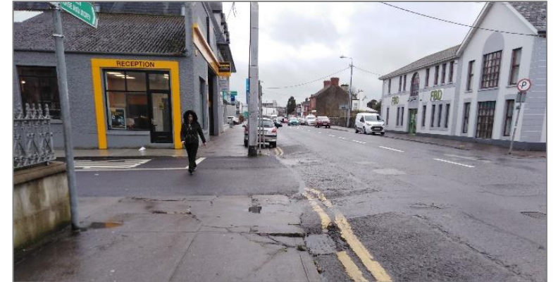
Poor pedestrian access across junction mouths with poor footway surface
