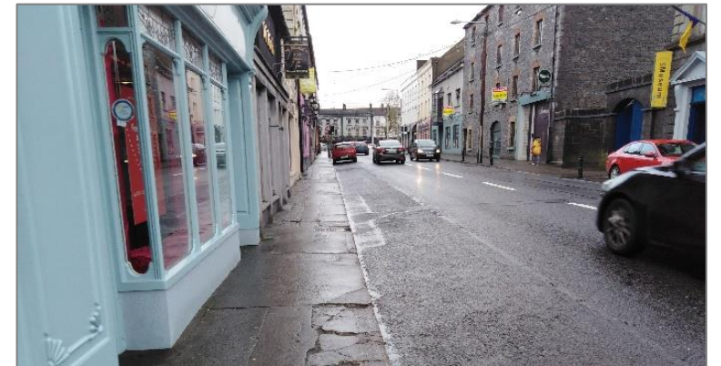
Footway deterioration due to vehicle overrun on existing narrow footways
