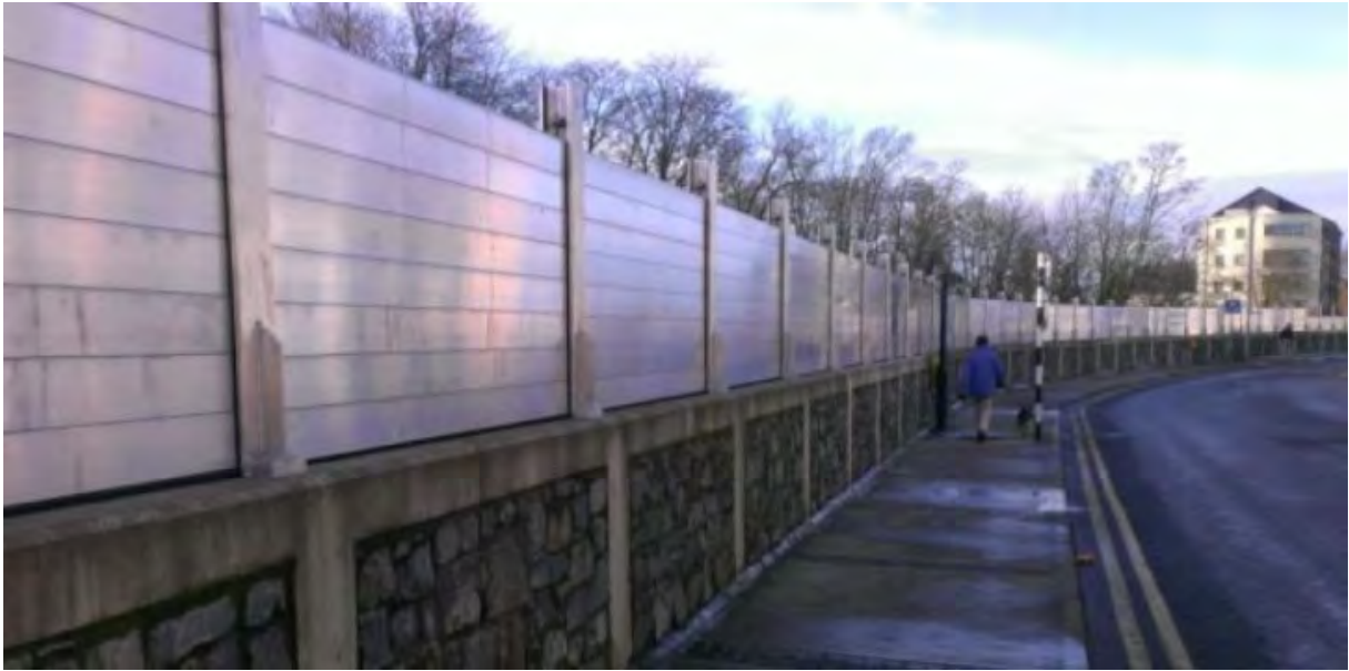
Figure 11-1: The Quays flood defence wall with demountable barrier system
