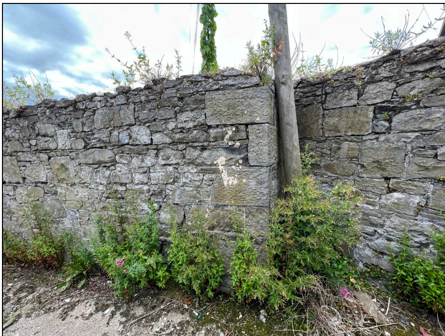
Plate 9: West facing view of the wall between the yard and the neighbouring building on Ashe Lane note the cur stone quoin stones.
