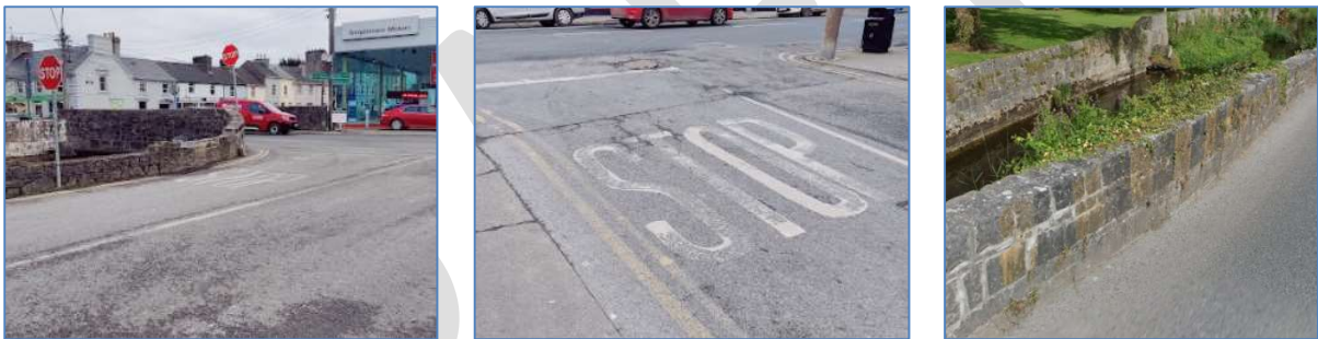
Figure 2-10 Faded Road Markings at the N62 / Blackcastle Road / The Mall Junction and Blackcastle Road
