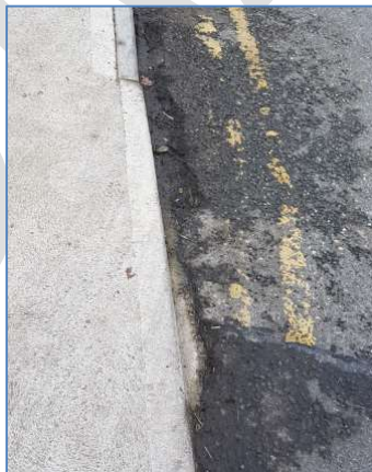
Figure 3-2 Trip hazards at drop kerb locations
