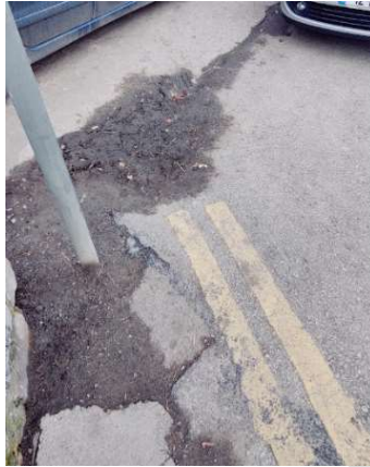
Figure 2-11 Area of Water Ponding on the East of the N62 / Blackcastle Road Junction
