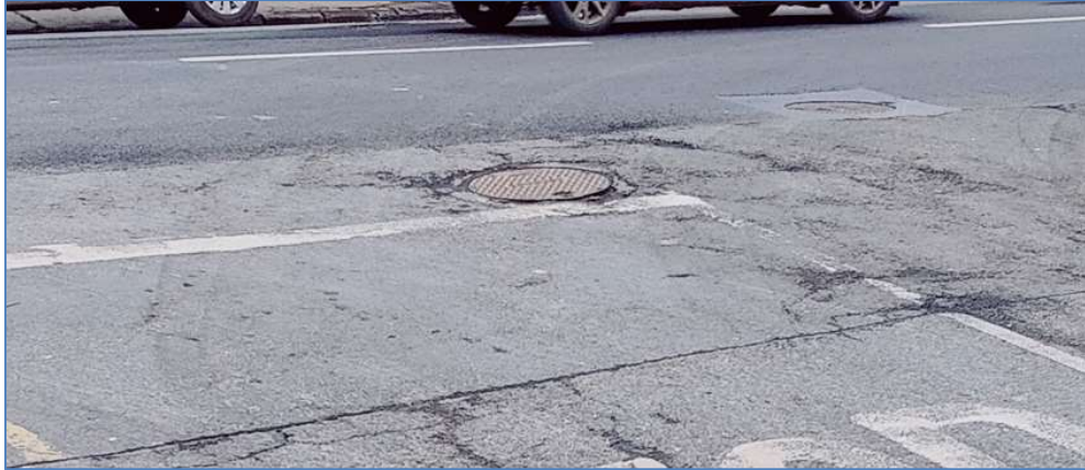
Figure 3-3 Pavement Deterioration at Utility Covers
