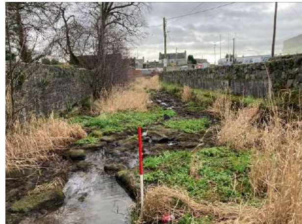
Plate 4 Walled Channel with overgrowth and bedrock exposed on base, facing south
