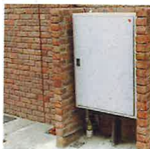
Six meter cabinet
