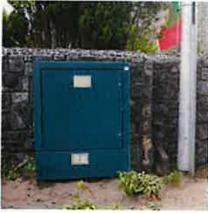
District Regulating Installation (DRI)
